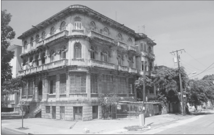
Many 1930s buildings, like this one in Havana, need renovation. Photo by Don Schneider.
